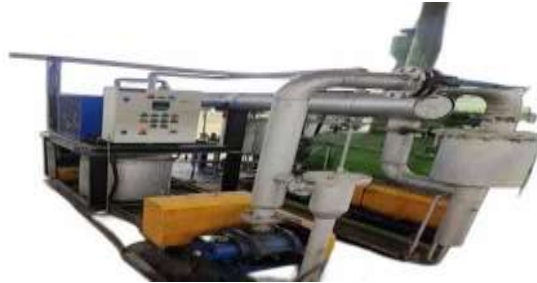
Figure 9: Biogas H 2 S Scrubber capacity
