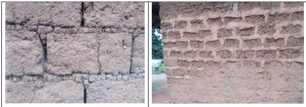
Fig. 1. CEB buildings damaged over time by environmental factors
