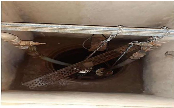
Fig. 3: Groundwater sump pit source
