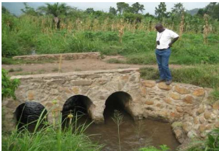
Fig. 5: Kanyampara Tripple Masonry Stone arch culvert, Span 4.2m built in 2012, Mukunyu Sub-county, Kasese District
