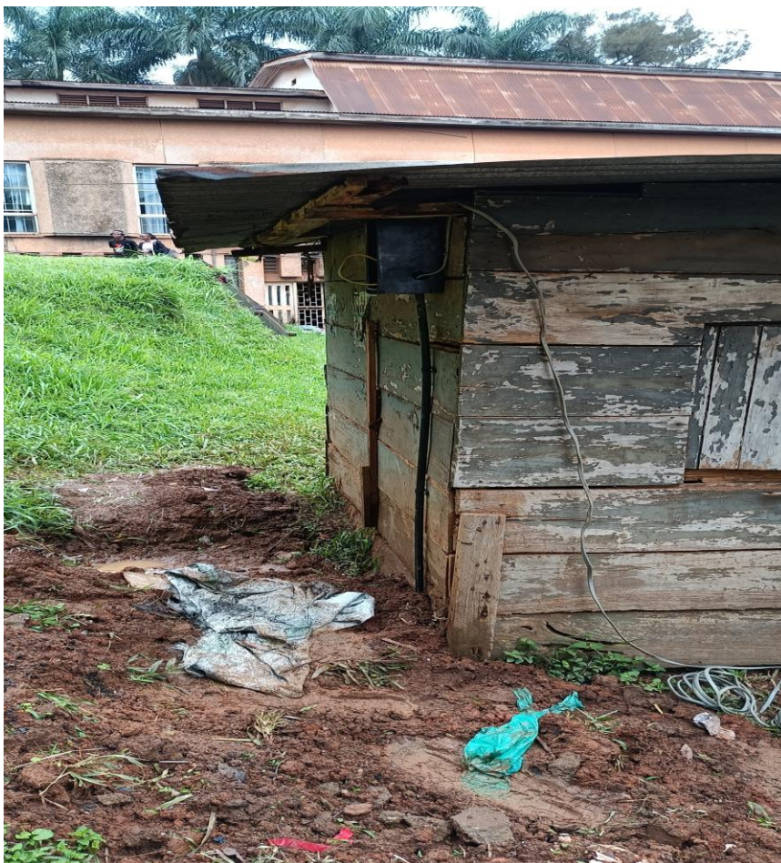
Fig. 1: Exterior view of the dilapidated kiosk used for wiring practice.
