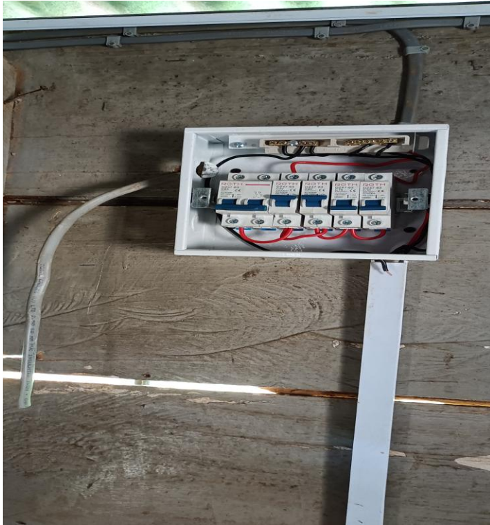
Fig. 2: Inside view showing loosely connected electrical accessories.
